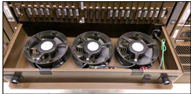
DMS-100 NTRX91AA FAN UNIT w/ EXISTING FANS
