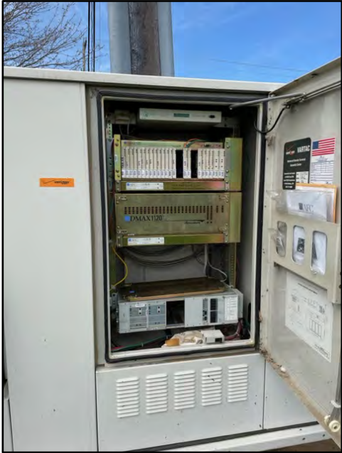
MESA BRIDGE CABINET (FRONT VIEW)
