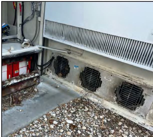
COMMSCOPE ALP 448/248 CABINET
