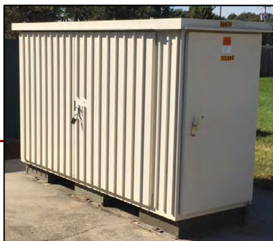
LS2000 CABINET (OUTSIDE VIEW)
