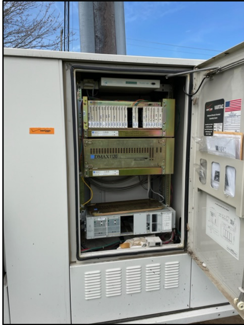
MESA BRIDGE CABINET (FRONT VIEW)
