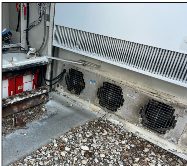
COMMSCOPE ALP 448/248 CABINET
