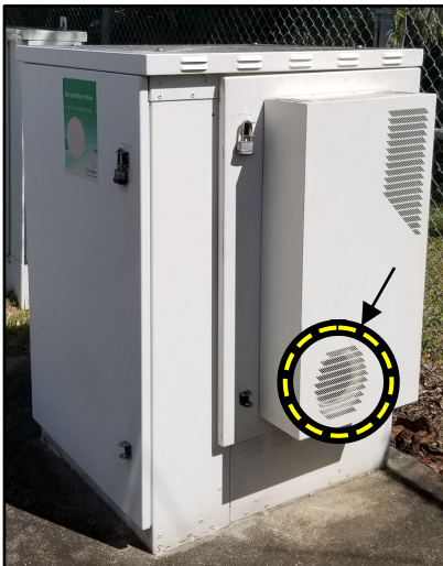
CALIX ODC-1000 CABINET (REAR VIEW)
