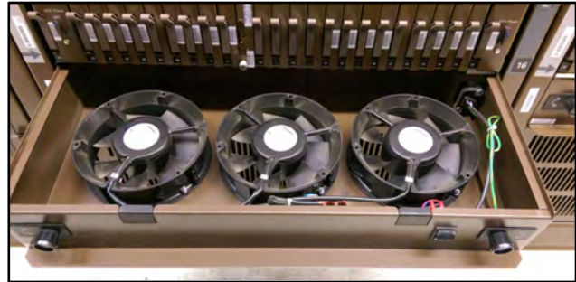
DMS-100 NTRX91AA FAN UNIT w/ EXISTING FANS
