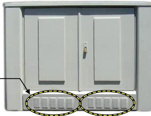
MESA 4 CABINET (FRONT VIEW)
